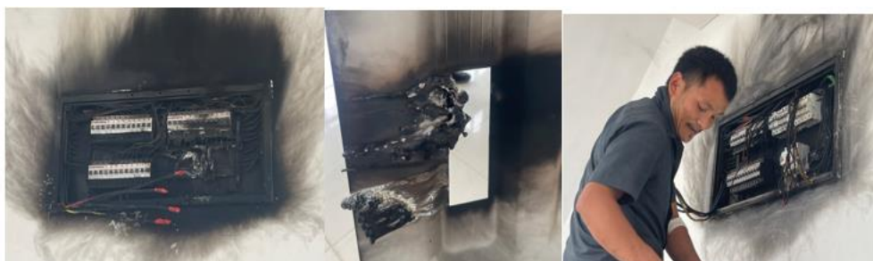
Fig 5. SMDB Burned due to Lightning Impulse.
