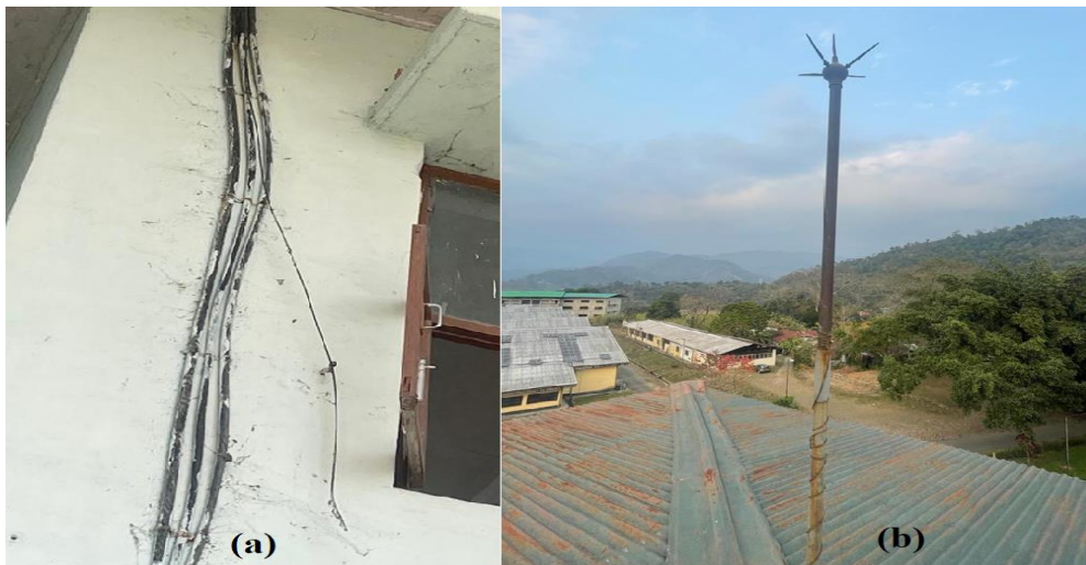
Fig 8. (a) Missing Down Conductors. (b). LA installed.
