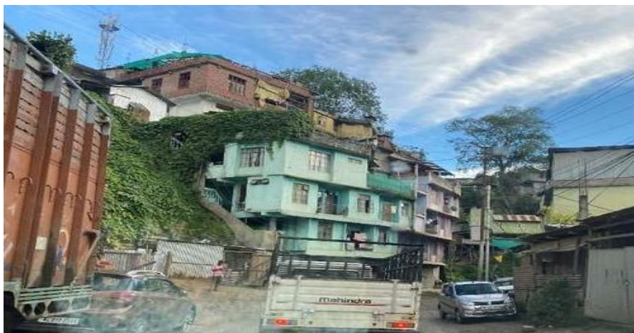
Fig. 3 Construction with no regard for slope stability
