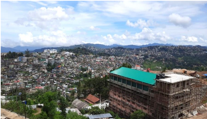
Fig. 1 High density development occurring in North-Eastern hill cities with no regard for the carrying capacity of hills
