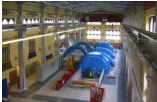
Figure 03: Powerhouse of the lower stage, 20x2 MW
